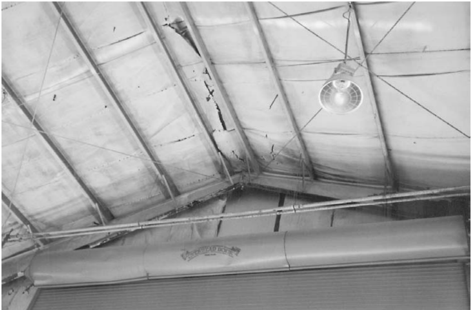
FIGURE 8.2 Cracked and torn vinyl vapor retarder.
